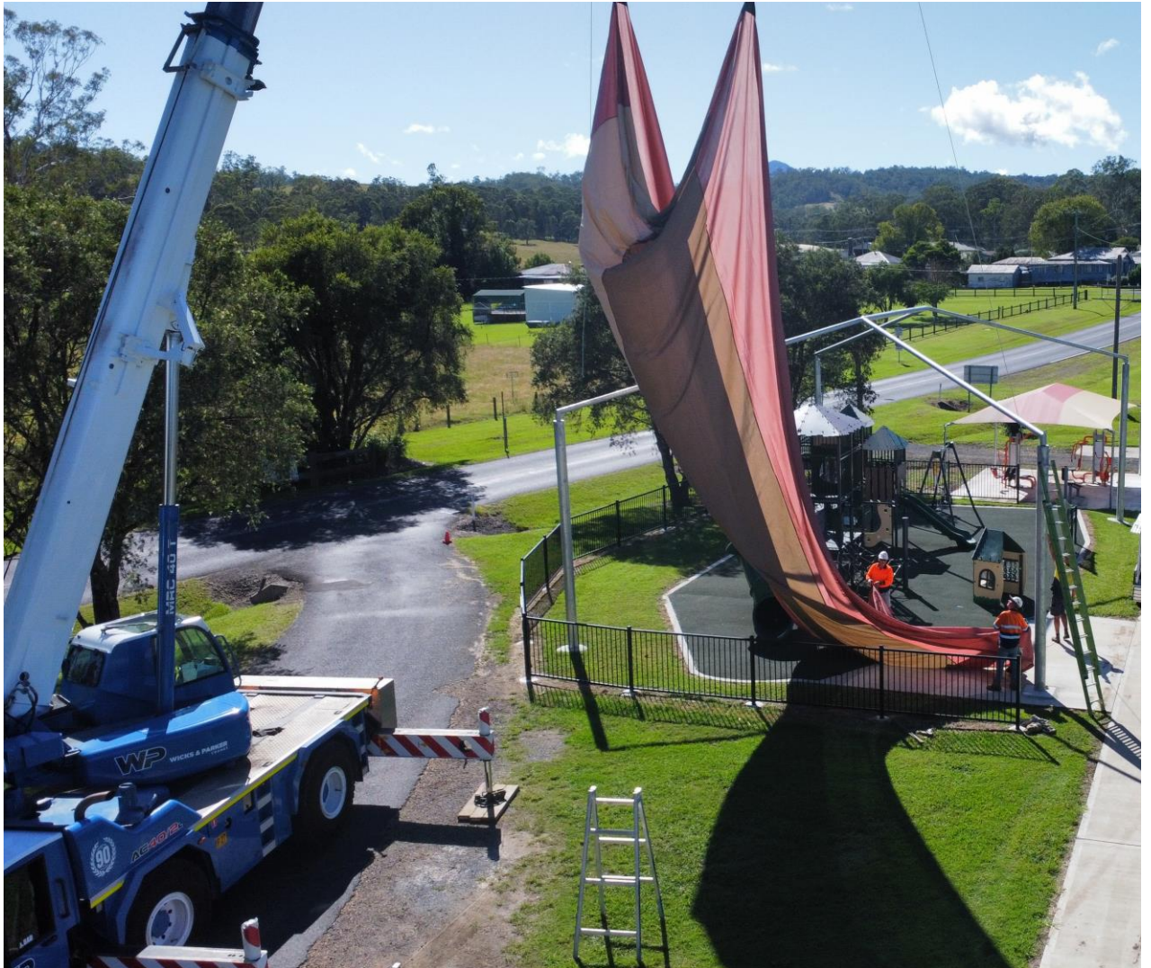
A new shade sail is installed over playground equipment at the Woodenbong Recreation Reserve.
