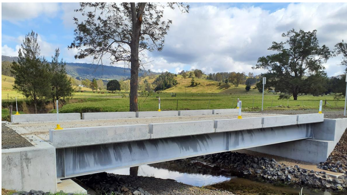
The Bingebeebebra Creek Bridge was one of 32 timber bridges Council replaced during the 2022-2023 financial year.
