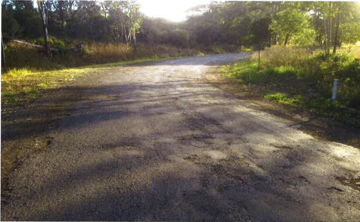
Photograph – Rough and Dangerous Pavement Surface
