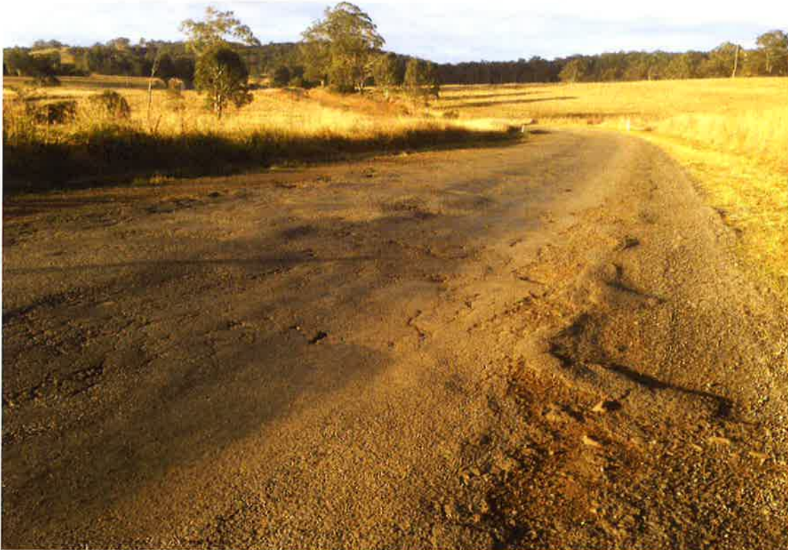
Photograph – Damaged Road Pavement
