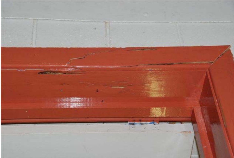
Photo 3.1 – White ant damage in door architrave
