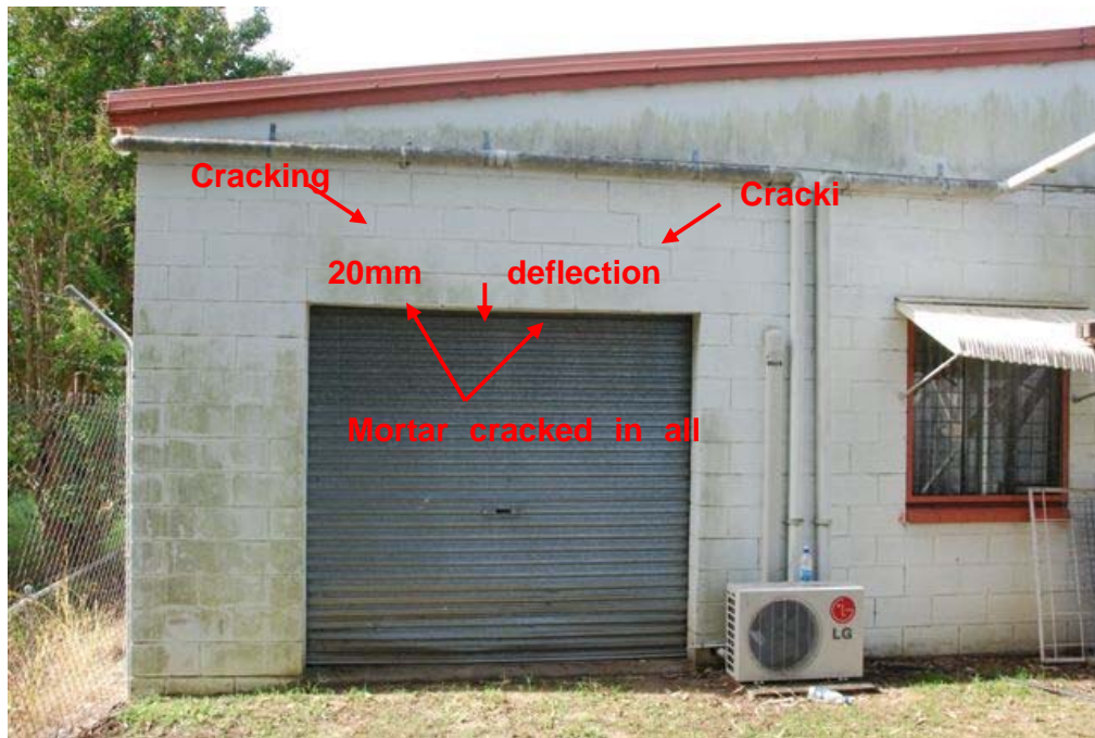
Photo 4.1 – Rear roller door indicating failure locations
