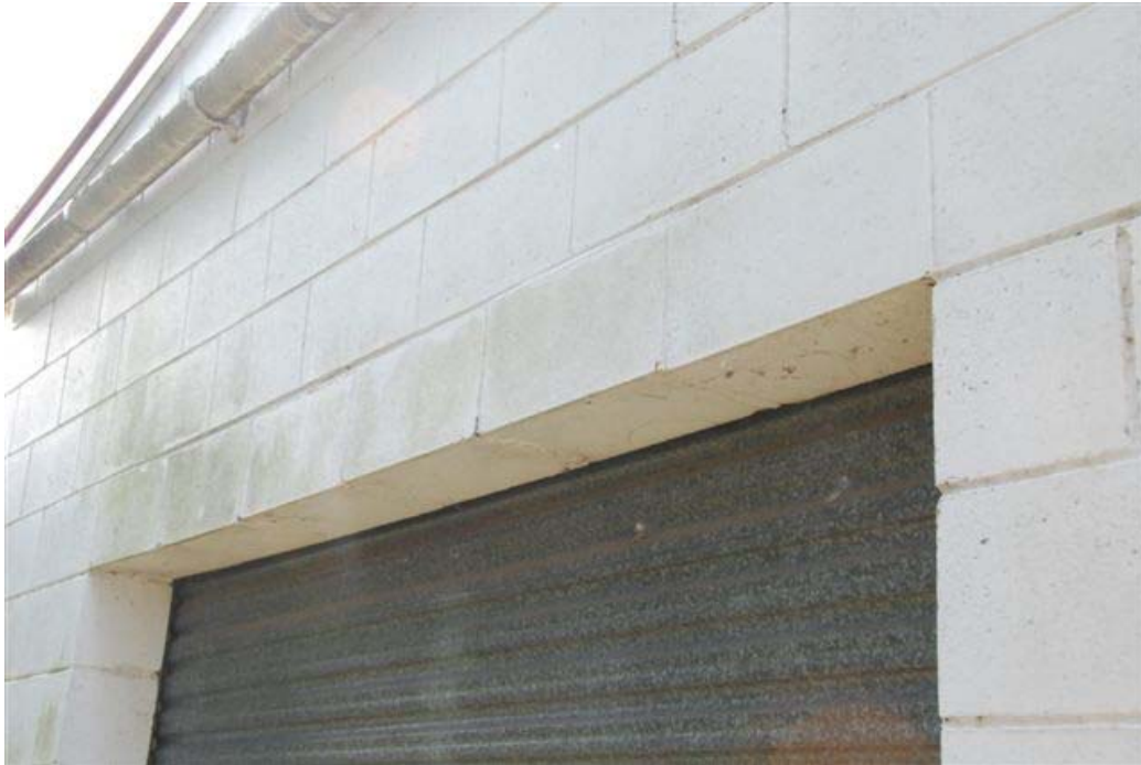
Photo 4.2 – Rear roller door indicating 20mm deflection and cracked mortar
