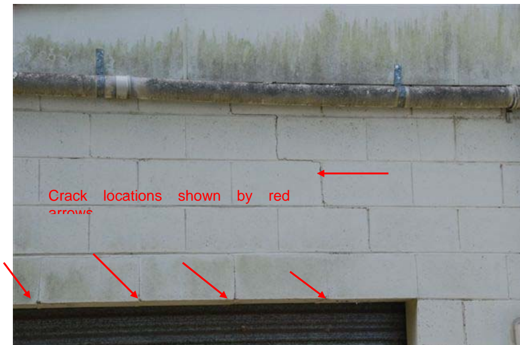
Photo 4.3 – Close up of rear roller door indicating cracked mortar
