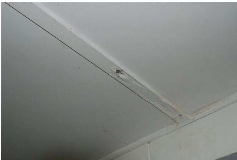
Photo 3.2 – White ant damage in ceiling cover strips
