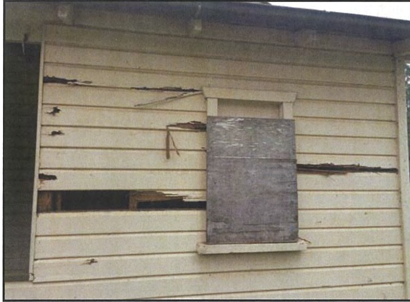
Section of Dilapidated Footings and External Lining
